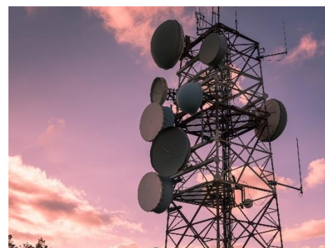
Image of a Radio Communications Tower
